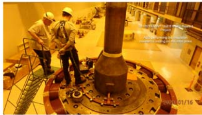
Figure 1: Final Insulation Resistance Testing on Rotor Poles
