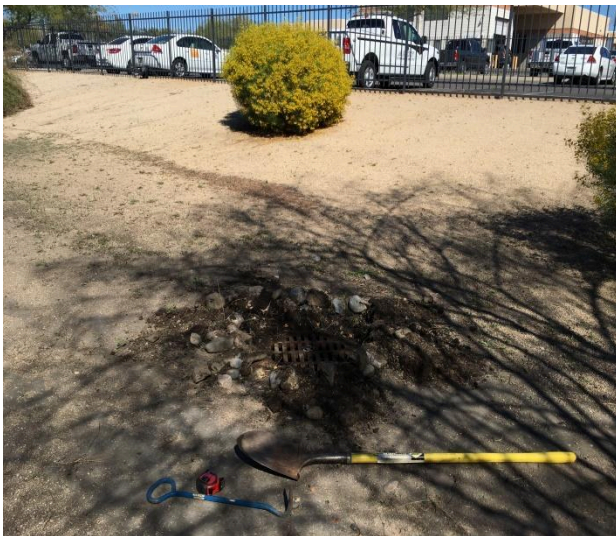
Figure 2- Sediment covering drywell inlet should be cleared
