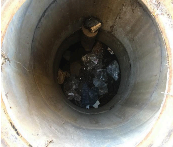
Figure 1- Debris accumulated inside a drywell should be removed
