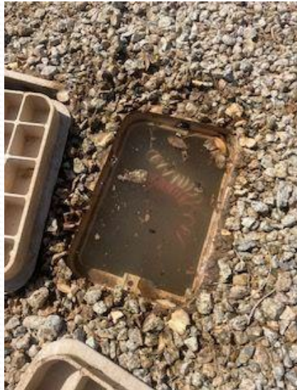
Flooded control box
