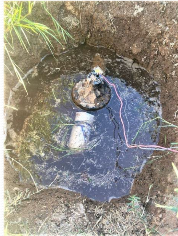
Leak at control valve
