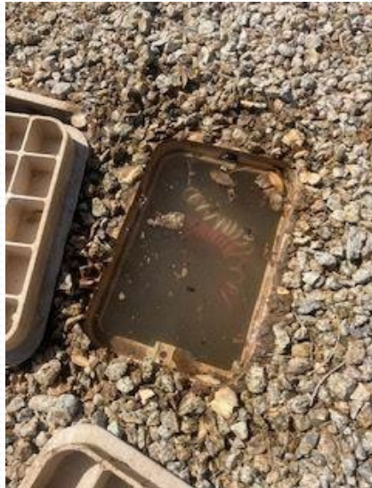
Flooded control box
