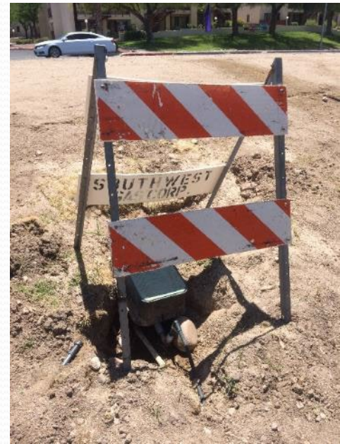
Underground leak near valve box
