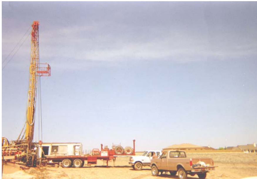
Figure 3 New Town of Prescott Valley well being drilled in the Lonesome Valley area
