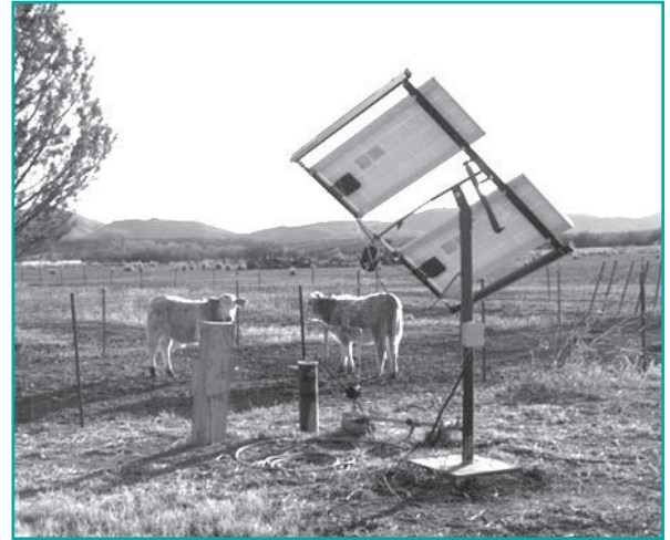
In rural Arizona, solar panels are commonly used to provide power to water supply wells where electric utilities are not available. Source: Richard Conway.
