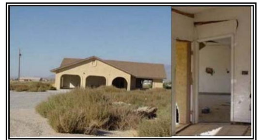
A House in Nevada Damaged by Land Subsidence and an Earth Fissure
